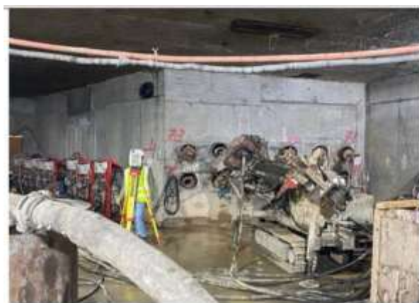
Figure 4. Horizontal directional drilling with annular space filling using mutual solution ( taken by the authors).
