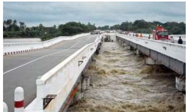
Fig. 1. A bridge along the Yangon-Mandalay highway is damaged by raging floodwaters in 2018.
